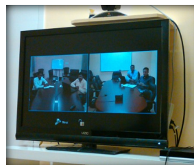
Video Conference Facility
